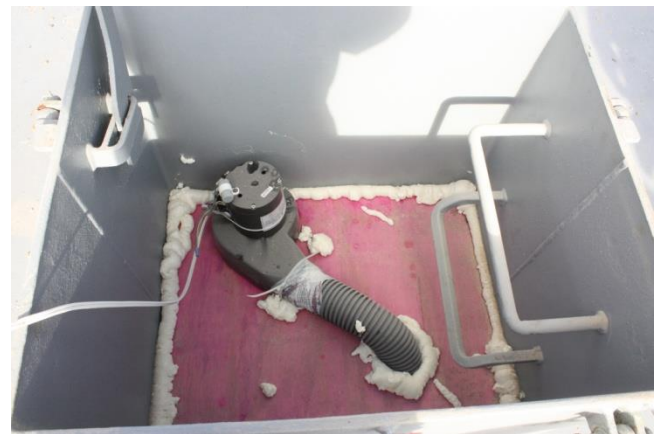
Recirculation fan positioned in hold access trunking
