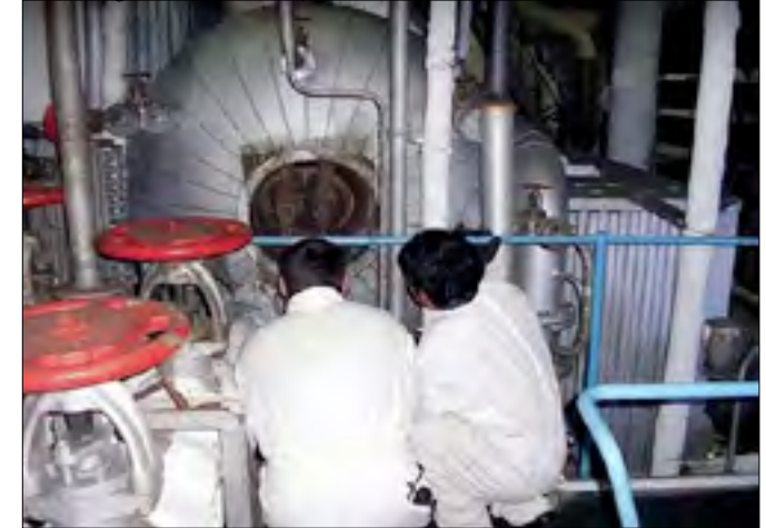
Examining the boiler that exploded
