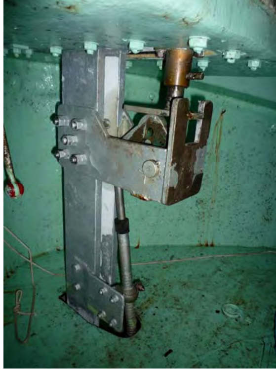
Photo 10: Underdeck Cam Plate visible for status check. Note this is incorrectly set.
